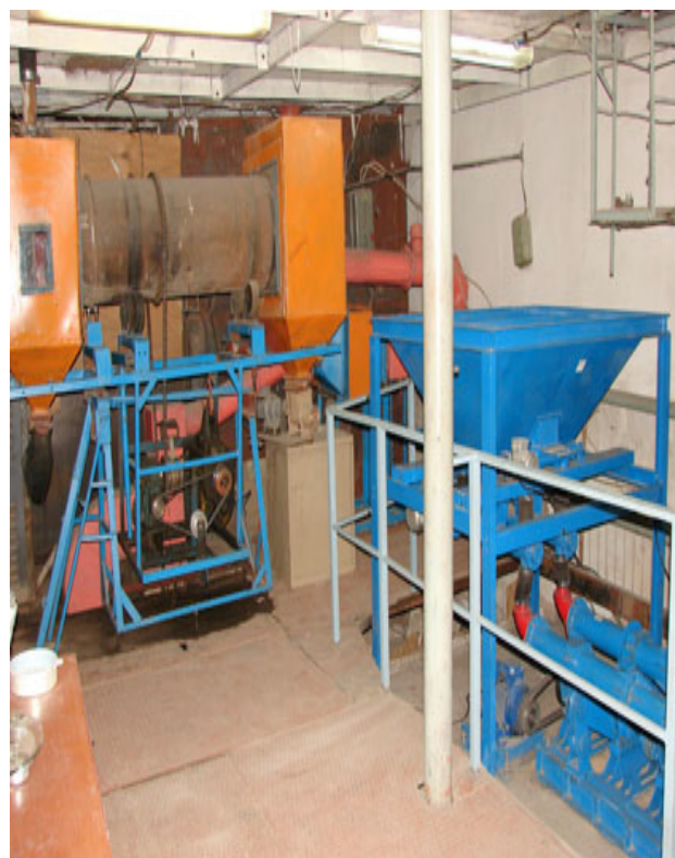
Figure 6: General view of the pilot plant.
